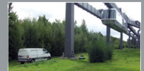
Ankerbolzenwartung und Messung der Restvorspannkraft Anchor bolt maintenance and measurement of the residual preload forces
